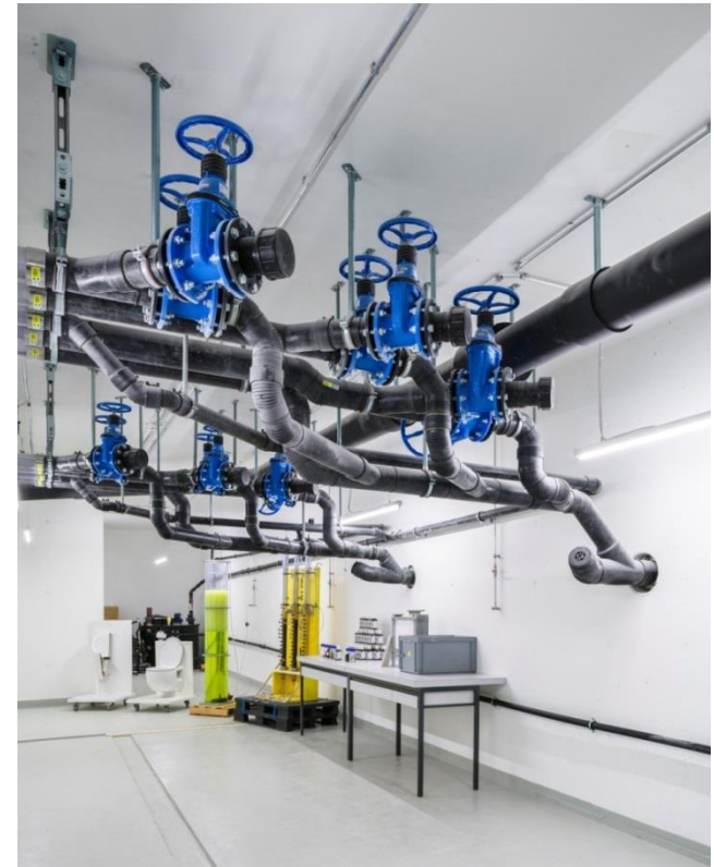
Separated wastewater streams entering NEST Water Hub laboratory
