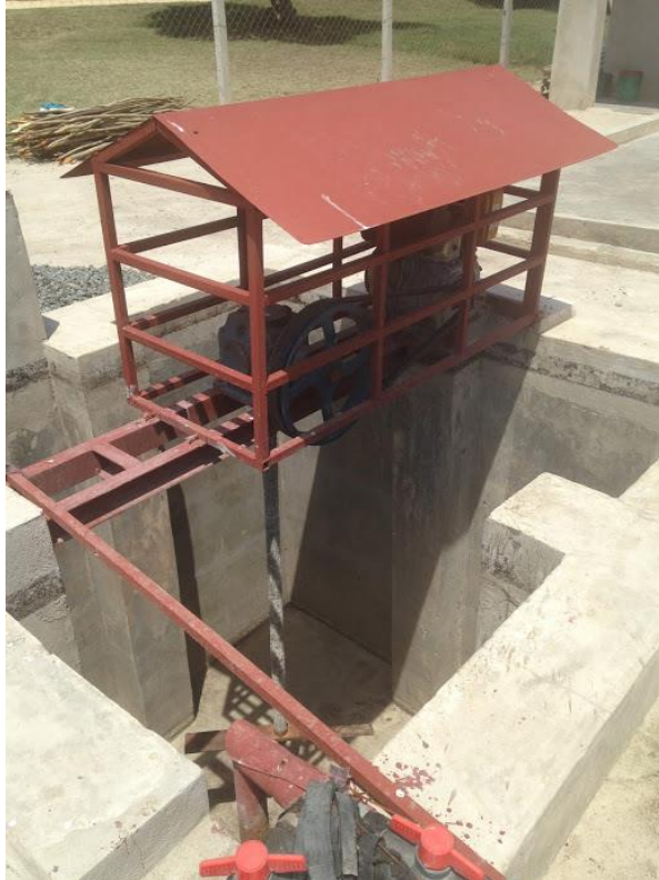
Conditioner mixing tank
