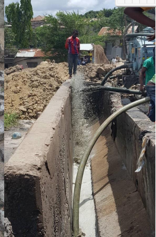
Vacuum trucks at Vingunguti stabilization ponds
