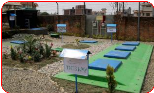
Faecal sludge reuse complex
