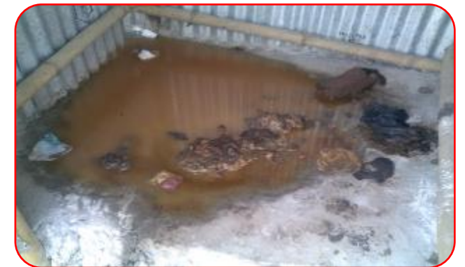
Overflowing toilets in campsites
