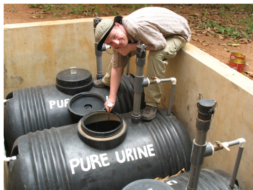
Urine collection tanks
