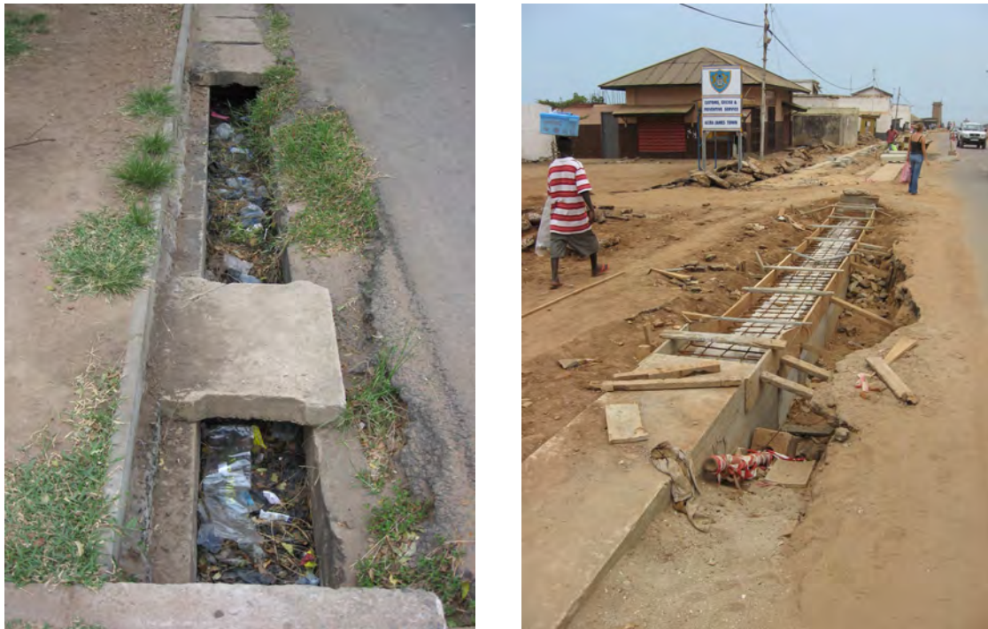
Figure 3.5: Drains blocked with rubbish and newly constructed covered drains in Accra
