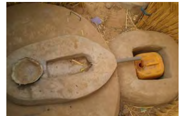
Figure 3. The composting latrine (Fossa Alterna) with urine diversion.
