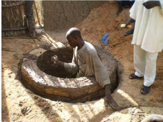
Construction of a composting latrine under supervision by the Rural Engineer of Aguié province
