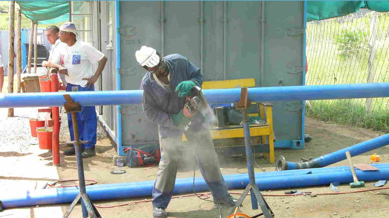
Work being done by a local contractor to water mains pipes at the Lower Maphephetheni site camp
