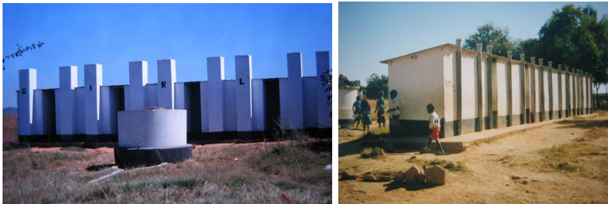
Blair multi-compartment Latrines were built at large numbers of schools. 10 cubicles were built together within a single structure. Many were built with hand washing facilities.
