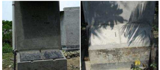
Fig. 12: Faeces vault doors originally steel, in the left picture, were later replaced in 2010 with concrete covers, in the right picture, due to corrosion (source: Antoine Delepière, 2009 (left) and Shahid Kamal, May 2011(right))
