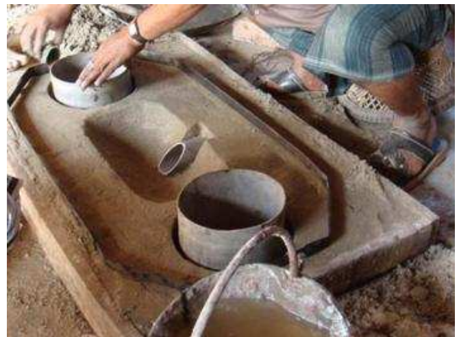
Fig. 6: Construction of a squatting pan by a local mason (source : Laxman Kharal Chetry, 2009).
