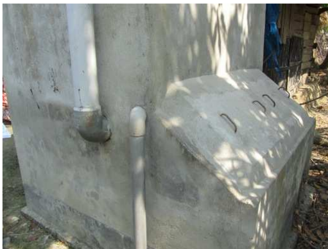
Fig. 9: The change in design of the faecal vault doors to concrete covers that took place during 2010 (source: Shahid Kamal, May 2011).
