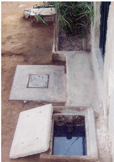
Photo 10: Grease trap chamber and household constructed wetland system. Housing Association, Los Topacios, Nievería, Lima
