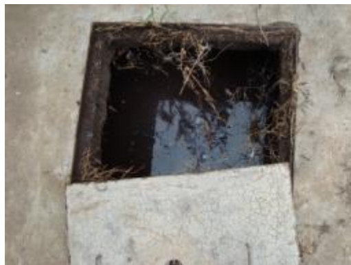
Figure 13: Filled up urine tank (source: L.Kraft, May 2011)
