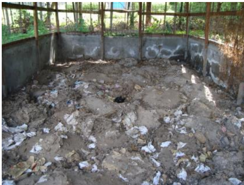
Figure 14: Dried faeces in the drying shed mixed with not degradable materials (Source: L.Kraft, May 2011)
