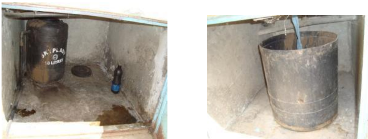
Figure 5: Left: Urine tank with small leakage in pipe Right: Container for faeces collection (source: L.Kraft, May 2011)
