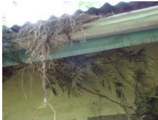
Figure 9: Blocked gutter for rainwater collection (source: L.Kraft, May 2011)
