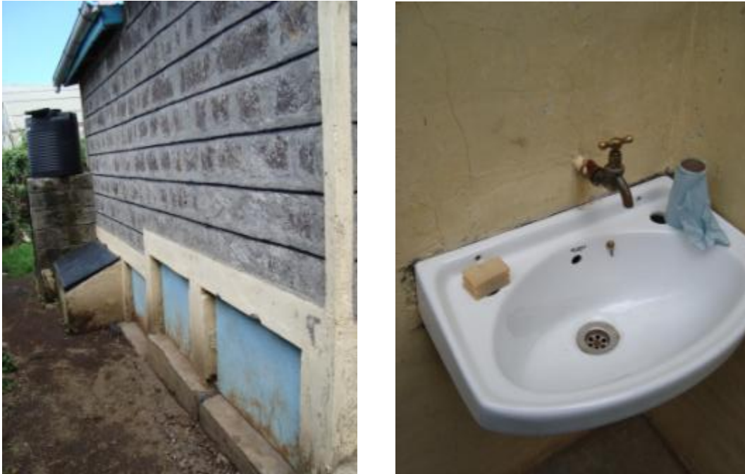
Figure 2 Left: Back view of UDDT facility with single chambers, double chambers and rainwater harvesting system Right: Handwash facility with soap and toilet paper (source: L.Kraft, May 2011)
