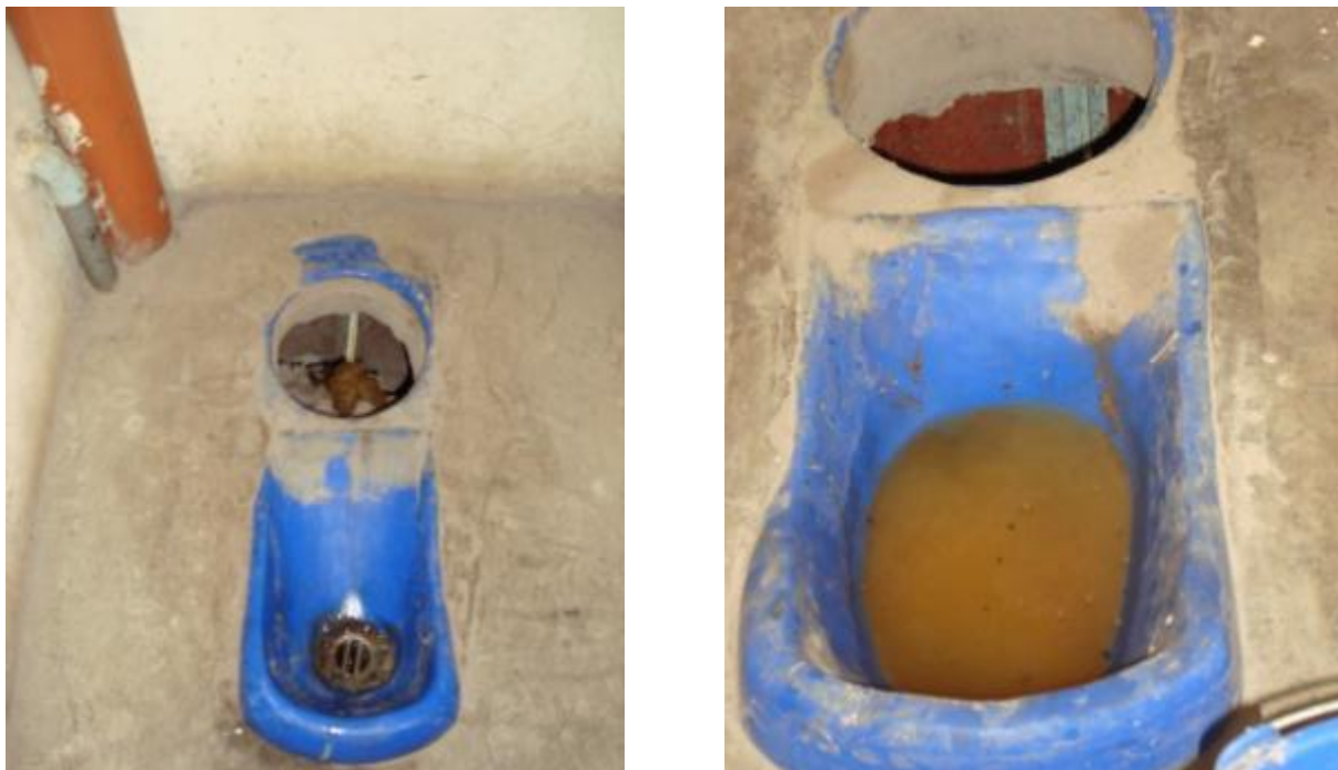
Figure 11: Left: Pilled up faeces are visible as containers are filled up signs of cross-contamination in the front part Right: Blocked urine pipe in the girls section (source: L.Kraft, May 2011)
