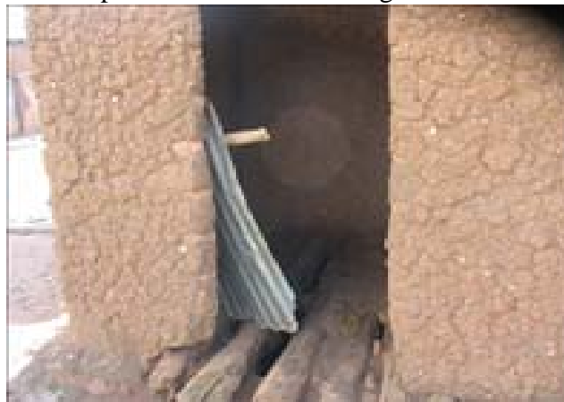
Figure 4-4: an example of a pit latrine in bad condition in Gitega sector (Sano, 2007)
