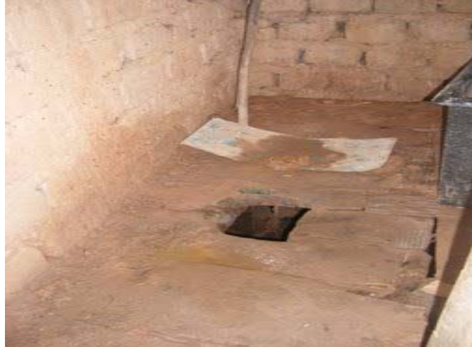
Figure 4-3: Private pit latrine at Gitega; an example of pit latrine with slab but bad smell. Though this toilet is covered by the slab, it smelt badly and was not clean. In the same sector, another pit latrine is shown in Figure 4-4 below:
