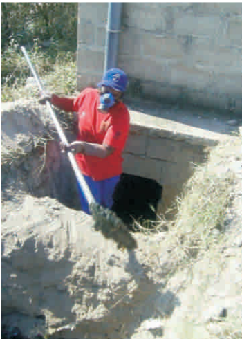
Figure 31: Waste is buried on site where space permits
