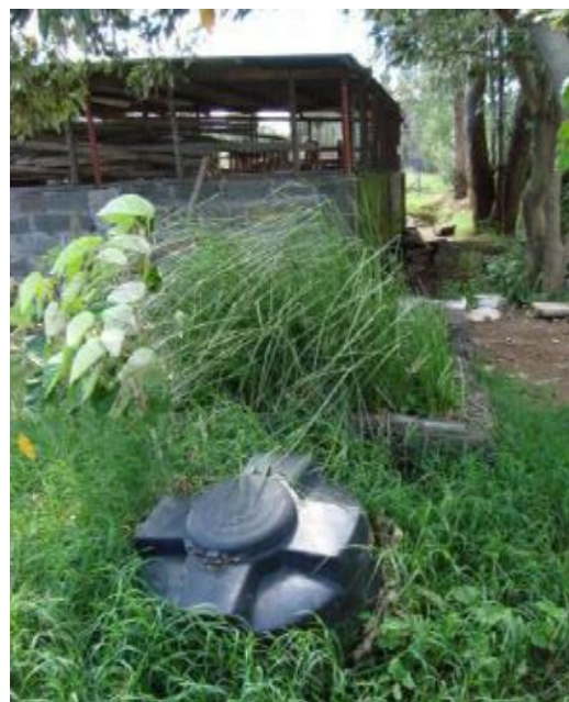
Figure 18 Greywater treatment system with settlement tank (Source: L.Kraft, May 2011)
