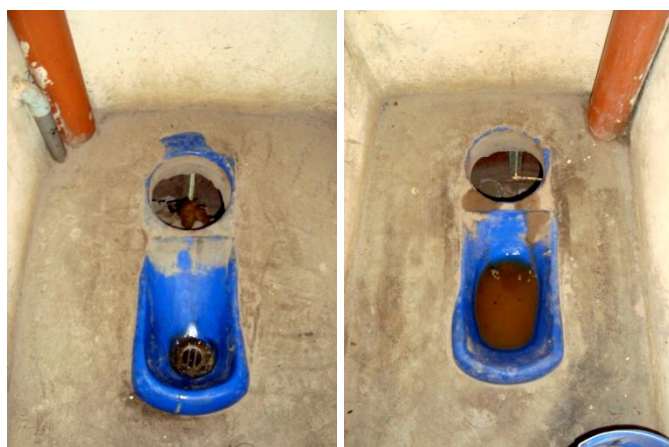
Figure 19 Left: In the boys section piled up faeces are visible as containers are filled up, fresh faeces are not covered with ash, signs of cross-contamination in the front part. Right: Blocked urine pipe in the girls section (Source: L.Kraft, May 2011)
