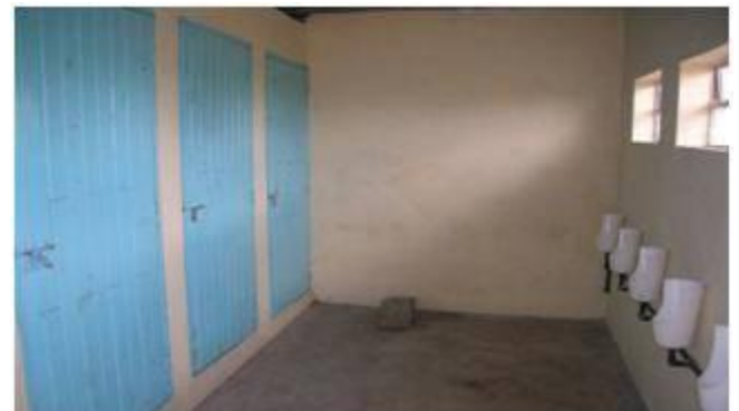
Figure 8 Inside the boys' toilet - 3 cubicles (left) and 6 waterless urinals (right) made of plastic buckets (Source: Muchiri, 2009)
