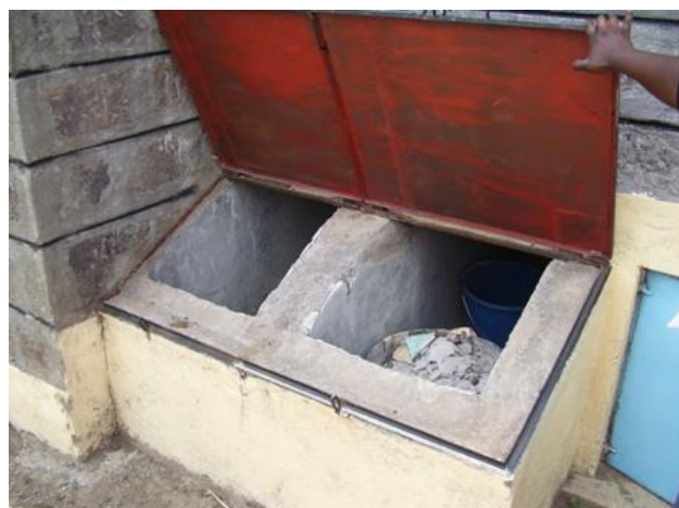
Figure 13 Containers are placed in the solar drier of the double vault compartment (Source: Steffen Blume, 2009)
