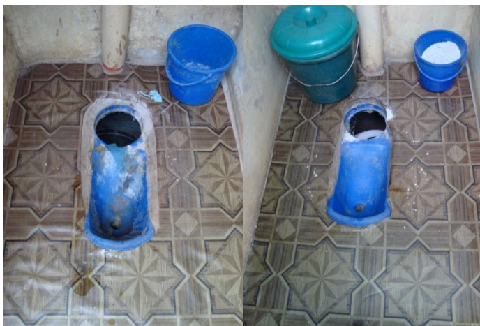
Figure 14 On the left, inside view of toilet used by men with empty ash container, urine on the floor and signs of faecal cross-contamination. Right: Inside view of toilet used by women (Source: L. Kraft, May 2011)
