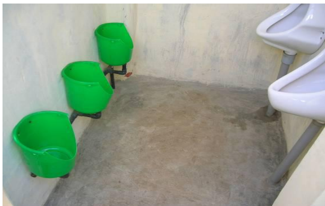
Figure 7 Inside the men's urinal showing the fabricated plastic containers urinal for the kids and standard ceramic urinals.
