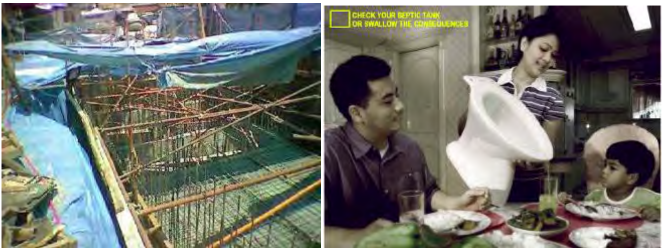
Figure 3. The Muntinlupa Market wastewater treatment plant under construction (left) and one of the IEC ads made by the project team as part of social outreach for the project (right)
