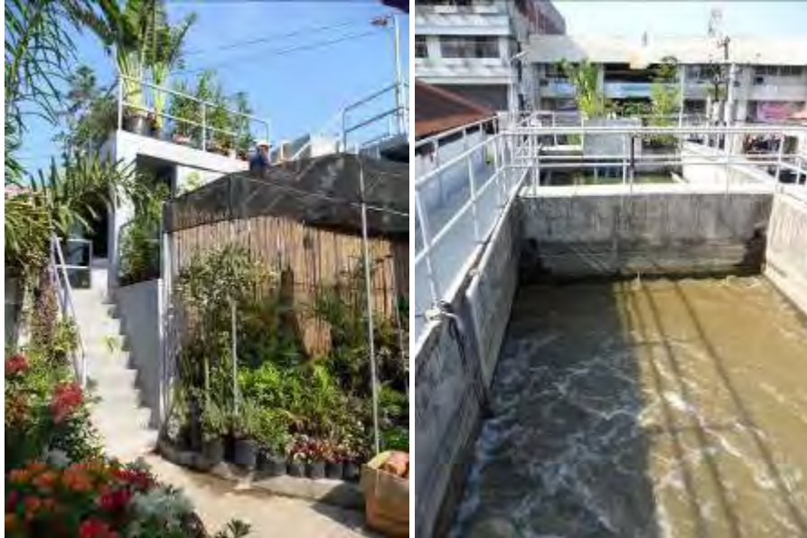
Figure 2. The San Fernando Market wastewater treatment plant (left) and its SBR and UASB (foreground/background, right)
