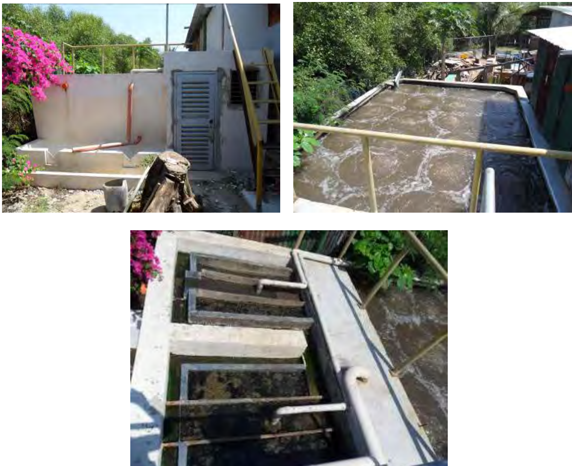
Figure 2. Photos of the LORMA WWTP showing: the side of the facility and the effluent discharge pipe to the river (top), the activated sludge pond (middle), and the clarifier (bottom)
