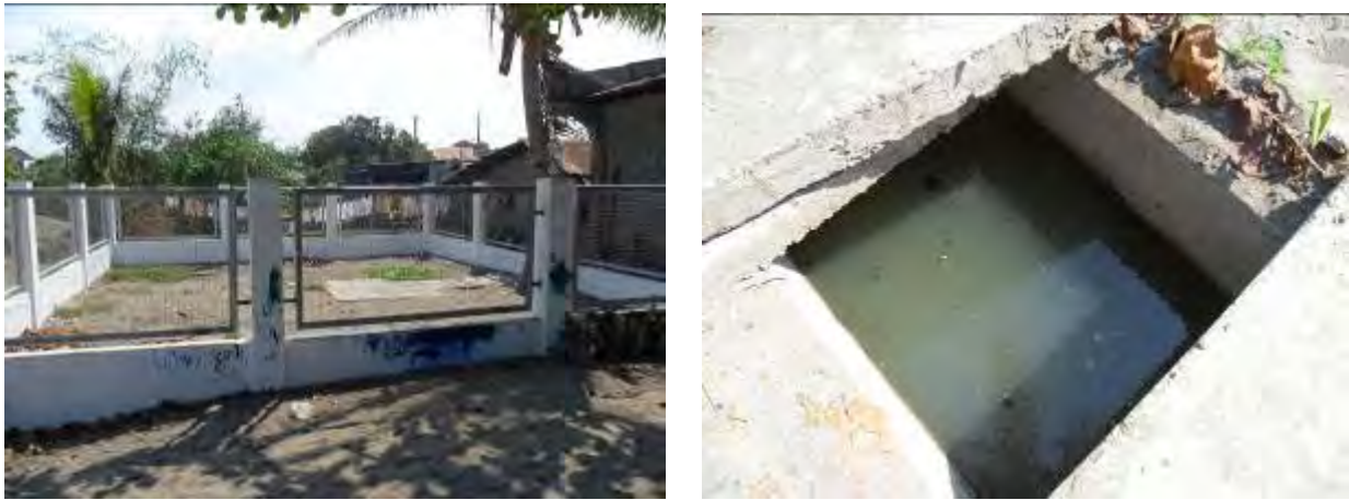
Figure 5. The completed Poro site (left) and a view inside the influent holding tank (right)
