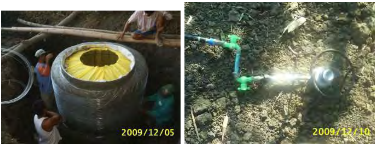
Figure 2. A photo of one of the biogas reactors under construction (left), and the simple gas burner used for its biogas (right) – made out of a pop can and some low cost plastic piping and valves
