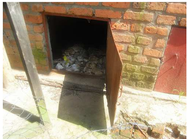
Fig. 10: Open vault of a UDDT in Kiziguro primary school. Paper is used as cleansing material.
