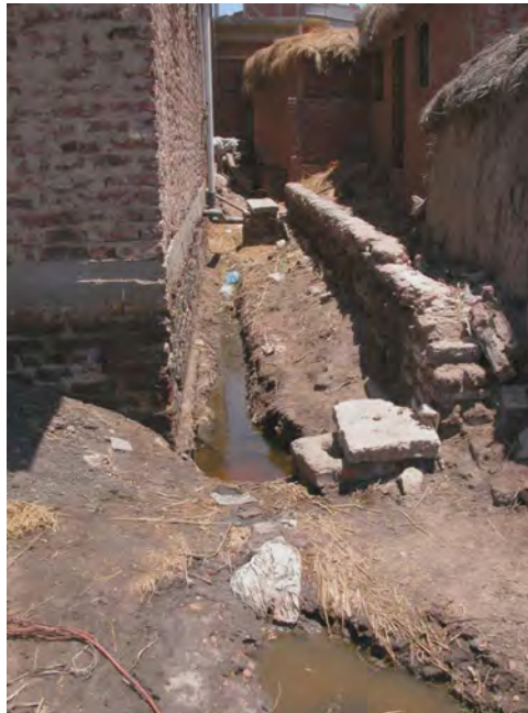
Fig. 7: Over spilling wastewater in El Moufty El Kobra (Sidi Salem district), Kafr El Sheikh Governorate, before implementation of a decentralised sanitation system (Source: GTZ)
