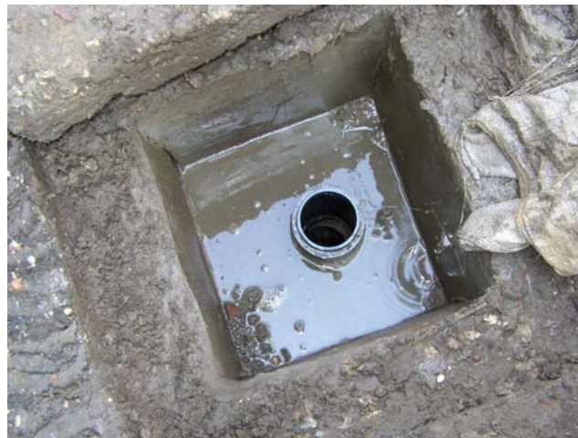
Figure 2. Clean-out chamber in the settled sewer network at El Mofty El Kobra
