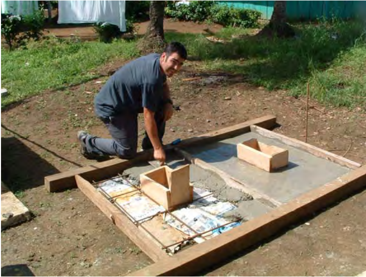
Figure 18. Construction of top floors of latrine showing wood forms to make seat holes *NOTE – Pieces or rebar, protruding upwards, can be placed in the floors at the corners to facilitate the construction of the housing structure later on (See Section 4.12).
