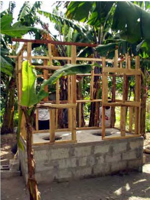
Figure 21 – Housing structure built over latrine chambers in Vanuatu, South Pacific. Concrete nails were used to connect the bottom wood beams to concrete floor. Source: Eric Tawney, PCV / Vanuatu and Master's International student
