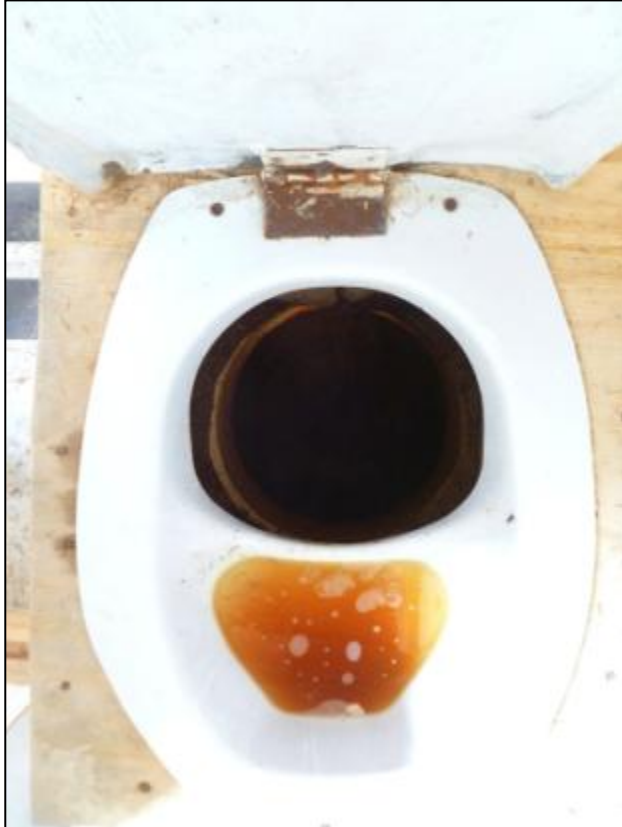
PHOTO BAD T1: SOIL UD toilet, blocked drainpipe.
