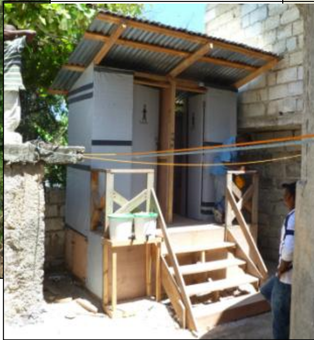
PHOTO T16b: GOOD positioning of SOIL UD toilet with just enough space for chamber access
