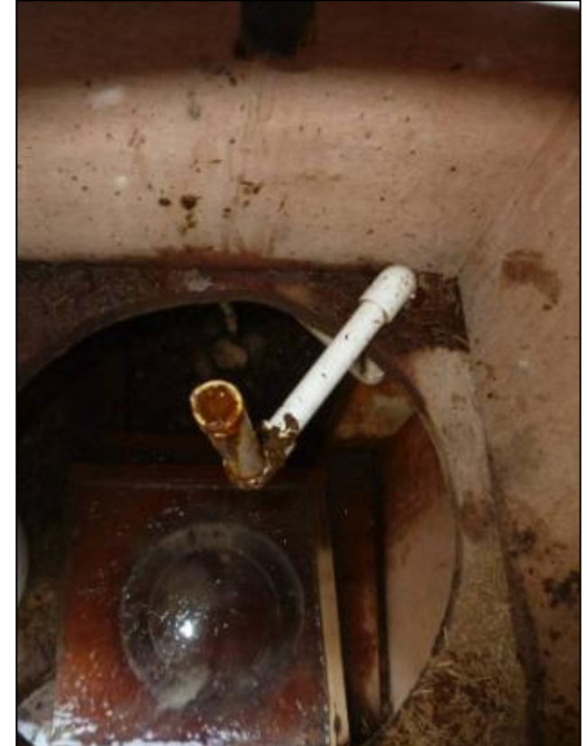
PHOTO BAD T3: SOIL UD toilet, detached drainpipe with urine spilling onto chamber floor.
