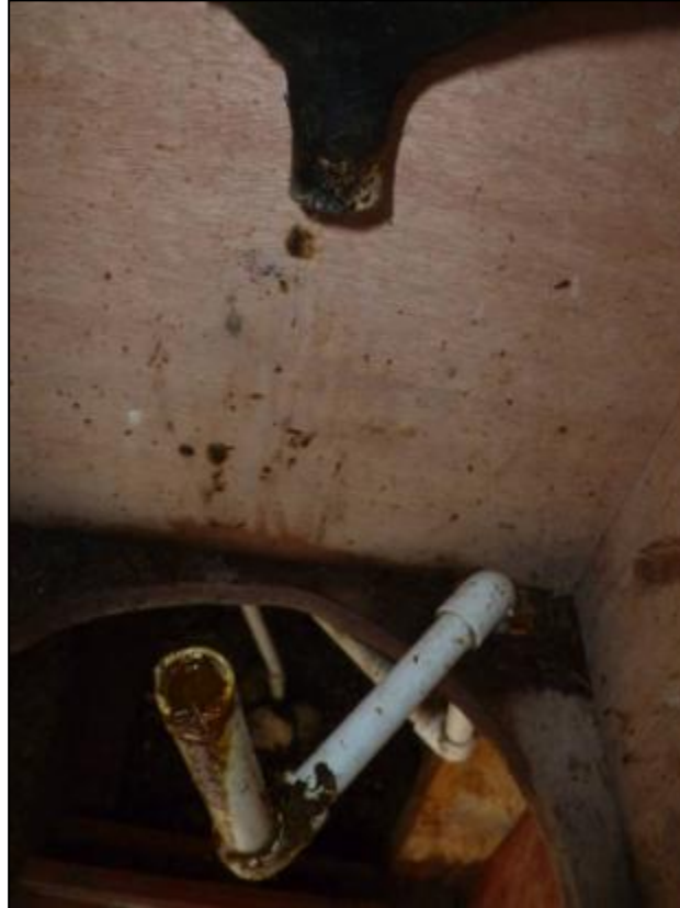
PHOTO BAD T2: SOIL UD toilet, blocked drainpipe detached from SOIL UD seat.
