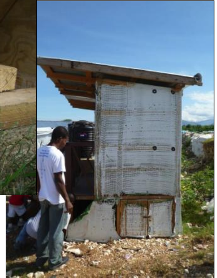
PHOTO BAD T9: Heat damage to plastic sheeting on side of SOIL UD toilet.
