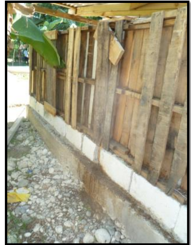
Photo K106: Jikaka leaking through block walls on outside of compost structure
