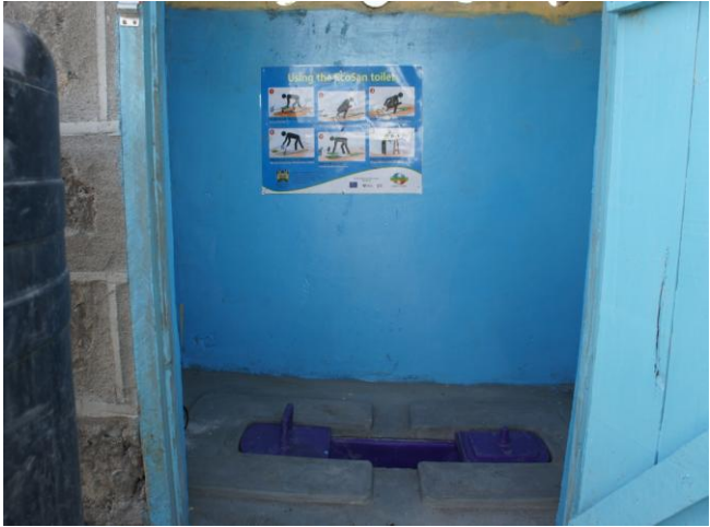
Interior of ecosan, chamber on left in use, sealed on right
