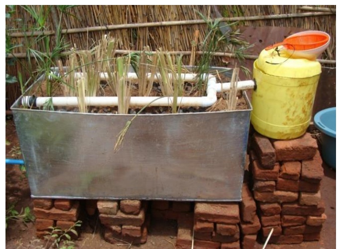
Fig. 3: The greywater treatment system after installation (source: A. Ilberg, 2010)
