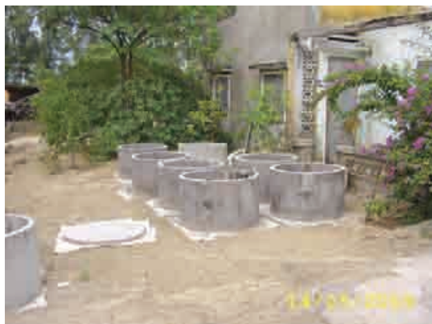
FIGURE 16: PRE-CAST RINGS FOR (SEMI) SEPTIC TANKS
