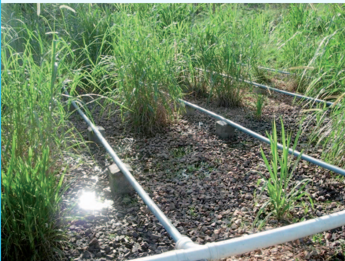
Figure 7. Constructed wetland at St. Franzis Naggalama Hospital.
