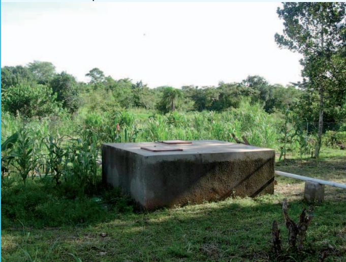
Figure 6. Mechanical pre-treatment of wastewater upstream secondary treatment in a constructed wetland.
