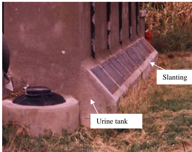
Figure 4.2a: Plate showing vaults of a solar dry toilet
