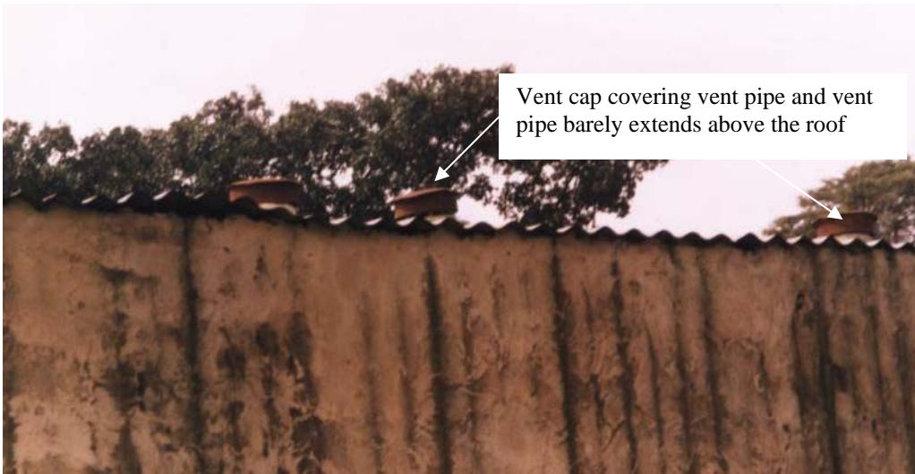
Figure 4.3: Plate showing Vent Pipes barely extending above the Roof
