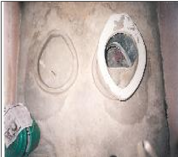
Photo 4-5: Sitting Ecosan toilet in two-vault toilet. To the left is blocked stance (K i 6)
