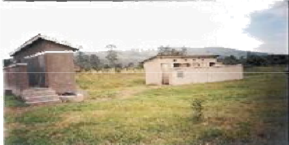
Photo 1-1: Kikungiri primary school, Kabale District where problems of use has forced children Nursery to P4 to use pit latrines whereas higher classes use the Ecosan toilet to the left
