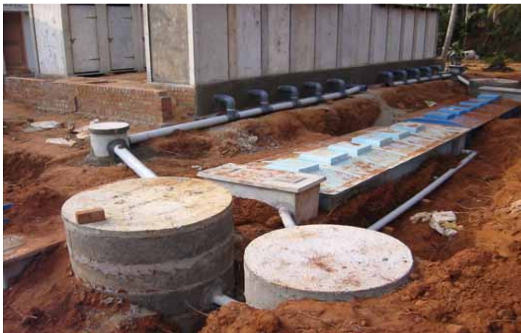
A prefabricated glass-fibre container DEWATS plant, with ferro-cement toilets installed after an earthquake in Indonesia.
