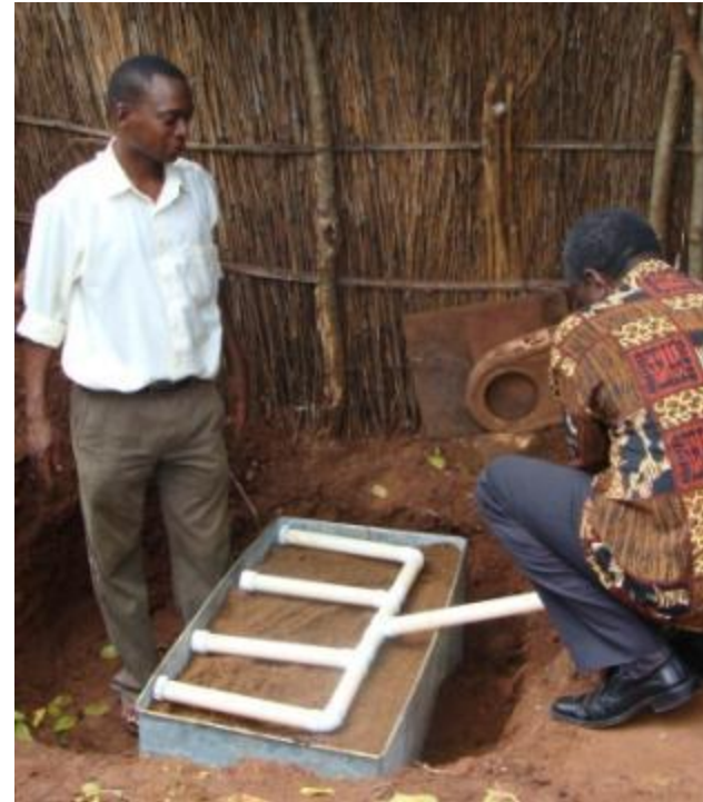
Perforated distribution pipes on surface.
