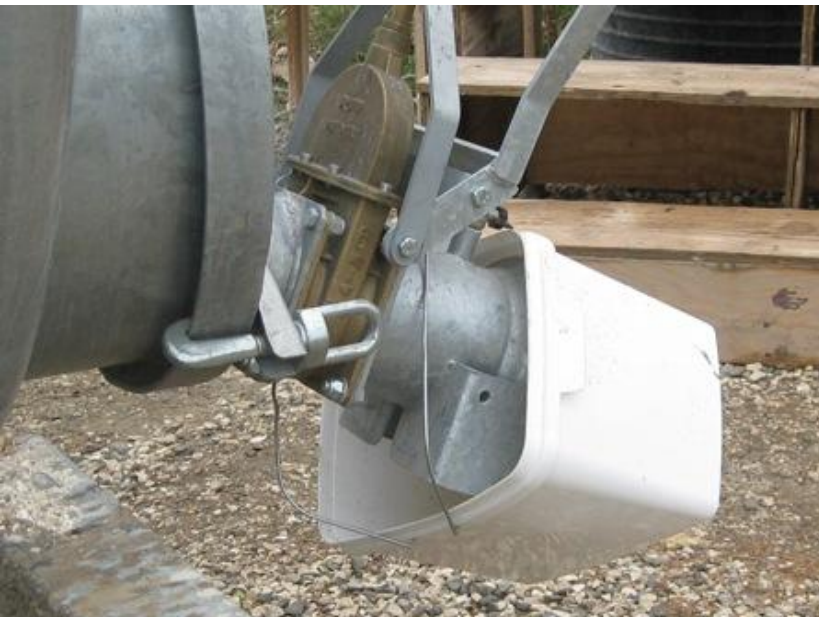
Protect from leaking valve
