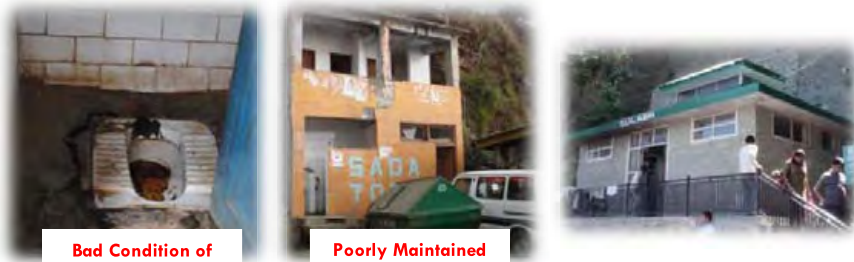
Bad Condition of Toilets
