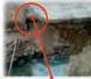
Discharge of blackwater into drains
