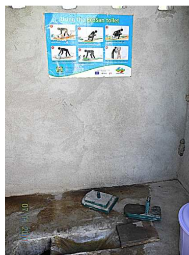
Figure 1. View inside a UDDT cubicle, at Kendu Muslim Secondary School with an explanatory poster on the wall, squatting pan with urinating hole and two holes for faeces leading to two vaults that are used alternately. In the right corner is a bucket for ash as dehydration material. The lids for the two faeces holes are also visible.
