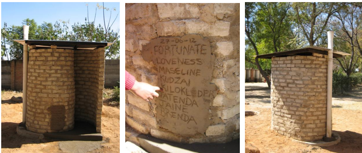
The completed toilet. The girls have great pride in building and carved their names in the cement plaque made on the front wall.
