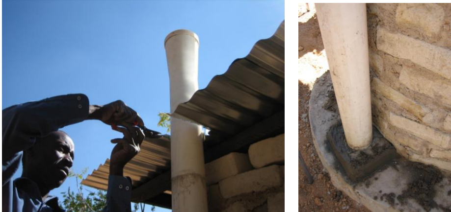
Cutting slot in tin roof for the vent pipe. The base of the pipe is fitted into the adaptor.
