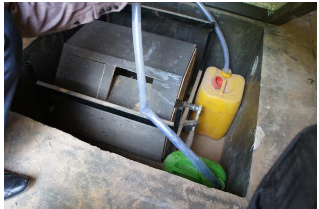
Figure 9. The composting reactor and tanks under the platform
