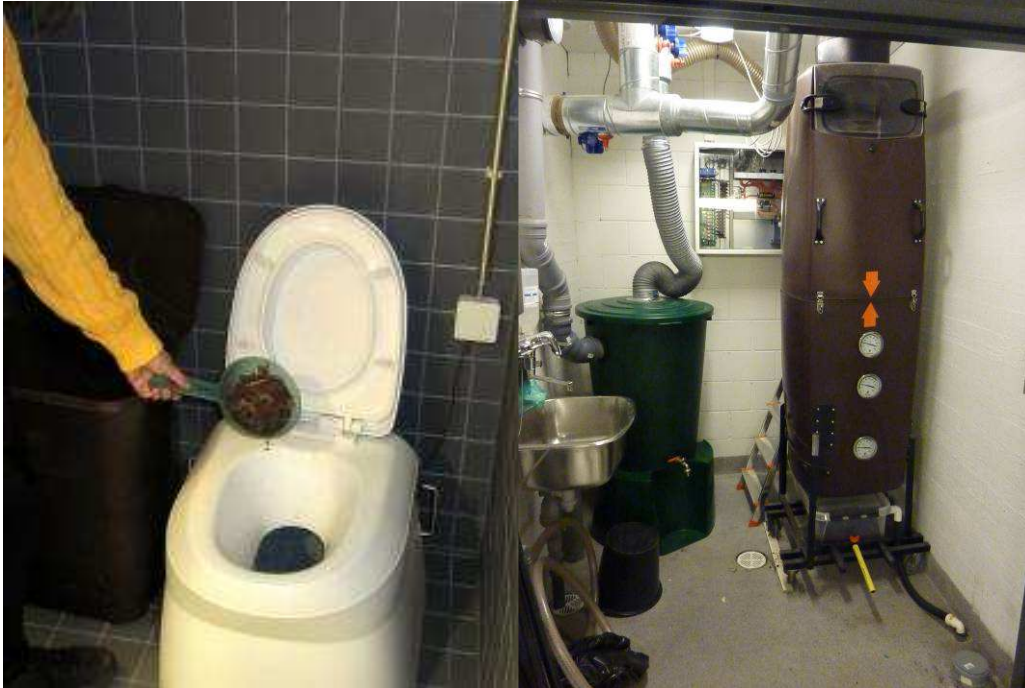
Figure 2. Two-story composting toilet seat in the first floor (left) and compost container in the basement (right).
