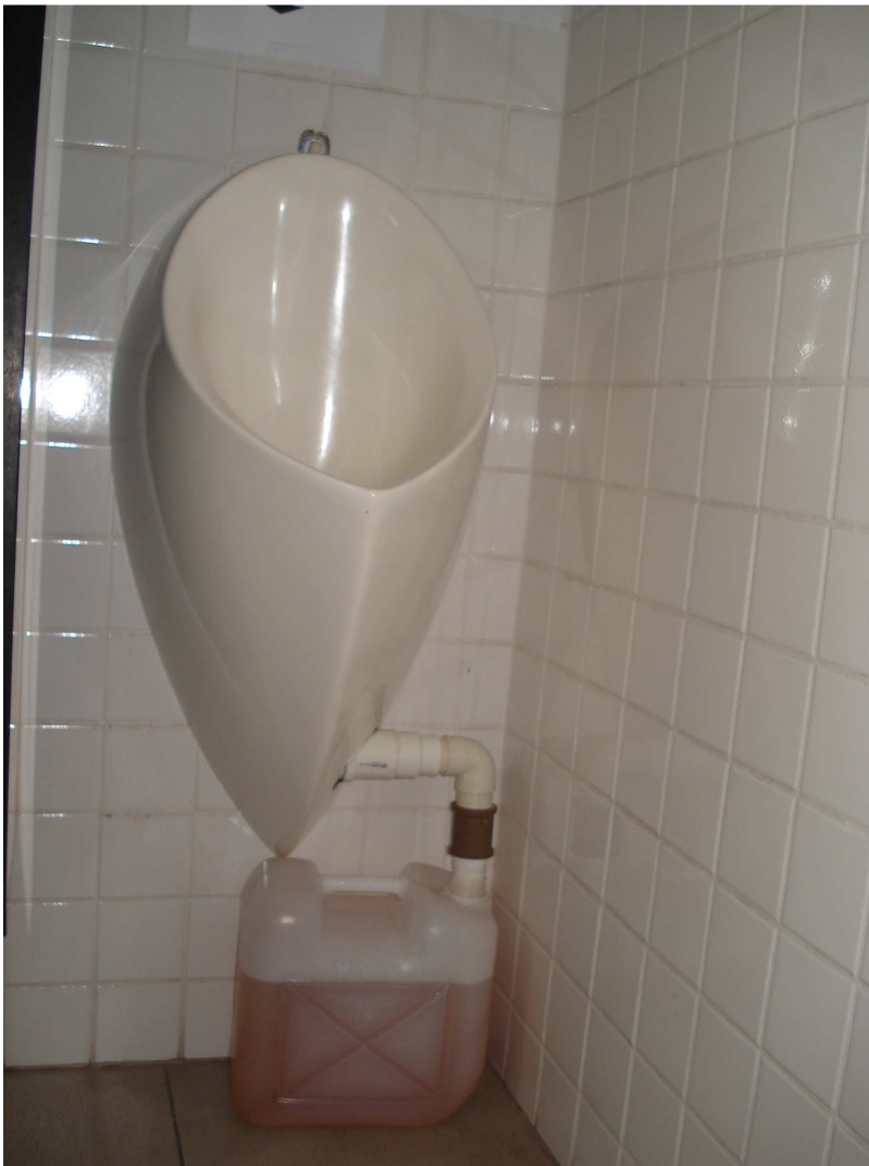
Figure 1- Waterless urinal installed in a male toilet in the campus .
