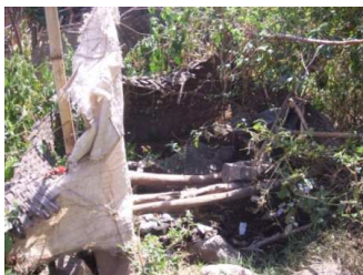
Figure: 1 : Typical pit latrines in Arba Minch. No proper floor, wall and roof
