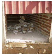
Figure: 23 UDDT vault in Arba Minch
