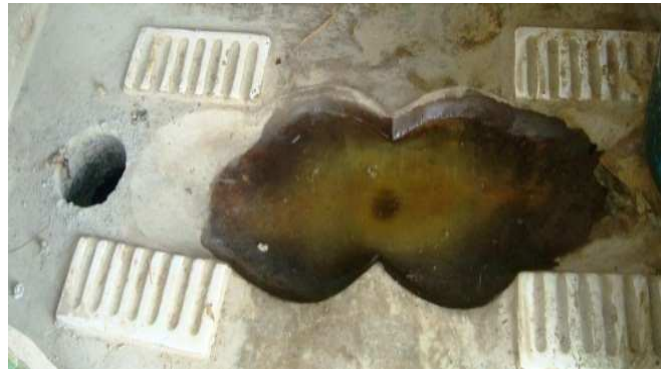
Figure 2 Urine pipe blocked at intervention area, Surkhet.
