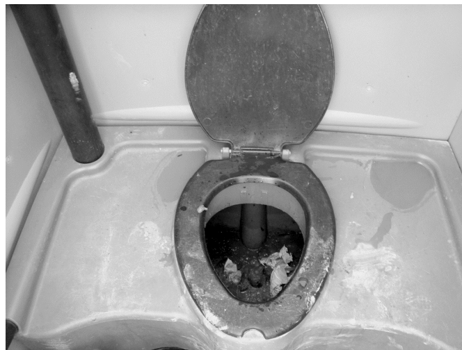
Figure 19: A portable toilet in Cite Soliel next to a medical clinic fills up and remains unattended. It is so unpleasant that the local children defecate openly on the ground around the toilets rather than go inside.
