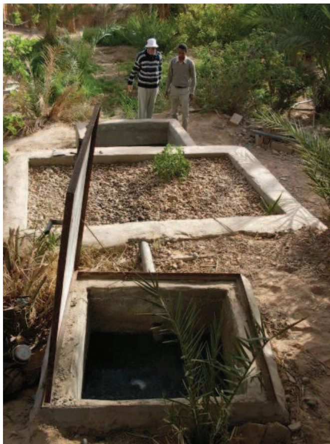
Fig. 8: The grease trap /settlement basin, filter and storage tank for the irrigation of the vegetable garden and the house of Mr. Boussouri (garden visible in the background) (source: AHT GROUP AG, 2011).
