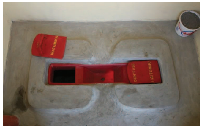
Fig. 8: Inside view of a UDDT with ash container on the right. The squatting pan has two faeces outlets: only the one on the left is currently in use. In the left corner is the ventilation pipe (not visible) (source: Moses Wakala, GTZ-Kenya, June 2008).
