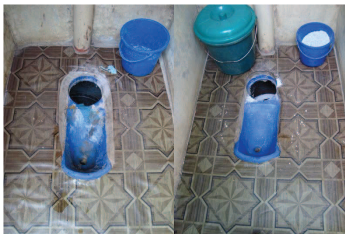
Fig. 14 On the left, inside view of toilet used by men with empty ash container, urine on the floor and signs of faecal cross-contamination. Right: Inside view of toilet used by women (Source: L. Kraft, May 2011)
