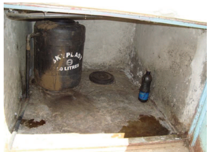
Fig. 12 50 liter urine tank with small leakage in pipe (L.Kraft, May 2011)
