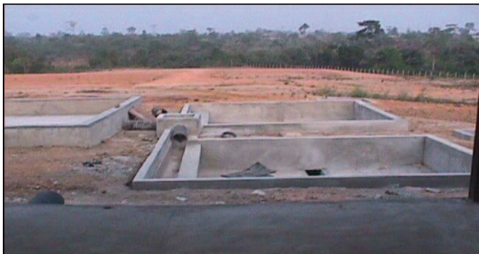
Fig. 4: Faecal sludge drying beds (source: Olufunke Cofie, 2002).
