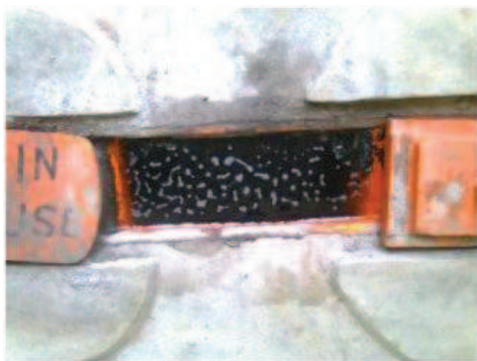
Fig. 14 A urine pipe of a urine diversion squatting pans got blocked with ash at Muslim Primary School, Mumias. Faeces drop holes are covered with lids on the left and right in this photo (source: Laura Kraft, GTZ, June 2010).
