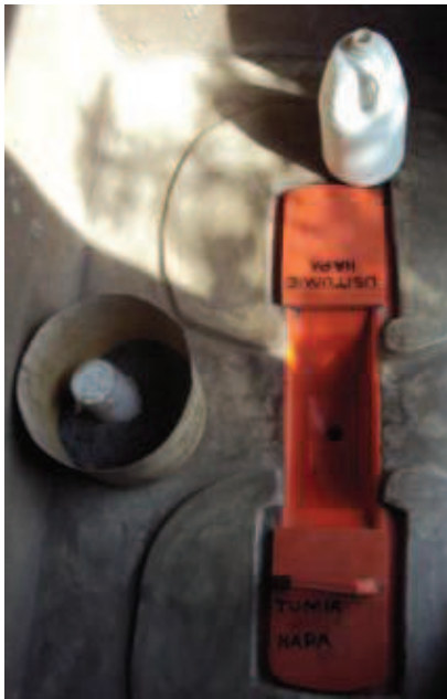
Fig. 7 Plastic urine diversion squatting pan with concrete footsteps inside a UDDT. Urine is collected in the centre; the two lids are covering the two faeces vaults (source: Laura Kraft, GTZ, June 2010).
