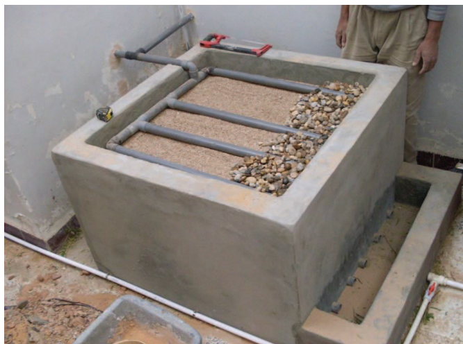
Fig. 7: Settled greywater is distributed across the surface of the filter medium using a series of perforated pipes (source: AHT GROUP AG, 2011)
