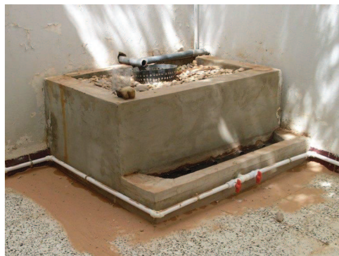
Fig. 4: The first pilot greywater filter and reuse system installed at the project offices (source: AHT GROUP AG, 2011).
