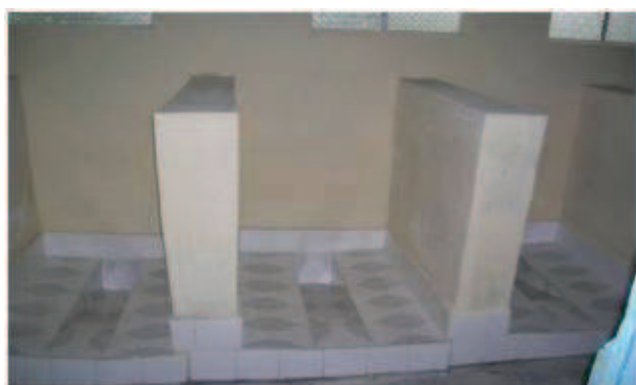
Figure 6 New waterless girls' urinals (squatting) inside the girls' toilet block (Source: Muchiri, 2009)
