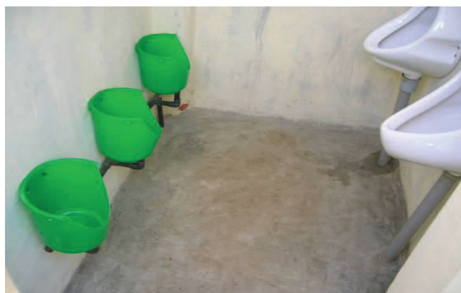
Fig. 7 Inside the men's urinal showing the fabricated plastic containers urinal for the kids and standard ceramic urinals.
