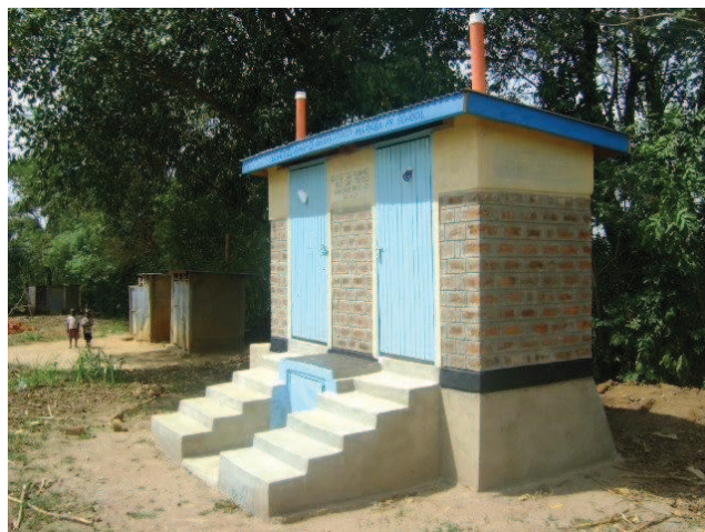
Fig. 5 Newly finished block of two school UDDTs in Western Province. Old pit latrines are visible in the background (source: Moses Wakala, GTZ, April 2009).
