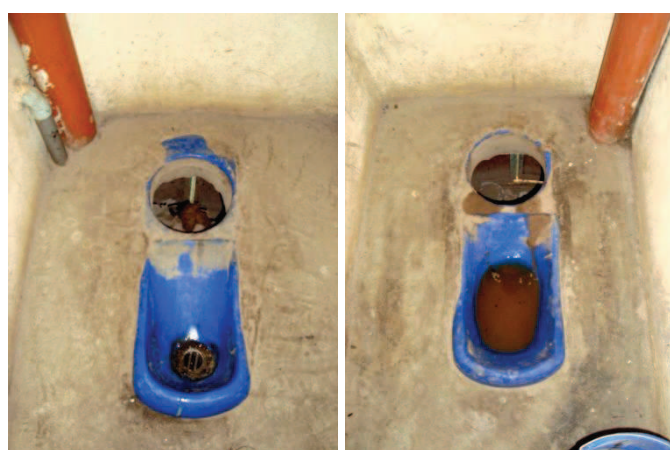
Figure 19 Left: In the boys section piled up faeces are visible as containers are filled up, fresh faeces are not covered with ash, signs of cross-contamination in the front part. Right: Blocked urine pipe in the girls section (Source: L.Kraft, May 2011)
