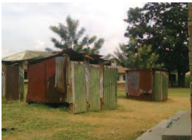
Fig. 4 Old pit latrines at Muslim Primary School, Mumias in Western Province (source: Laura Kraft, GTZ, June 2010).
