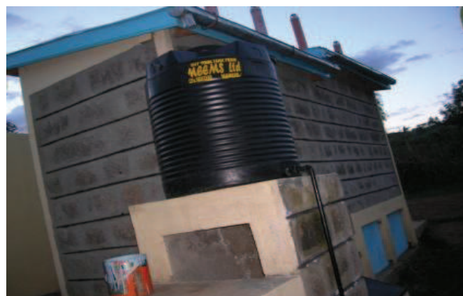
Fig. 8 Roof water harvesting system for hand washing at the new UDDT.
