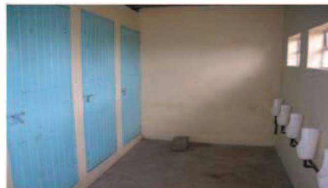
Figure 8 Inside the boys' toilet - 3 cubicles (left) and 6 waterless urinals (right) made of plastic buckets (Source: Muchiri, 2009)
