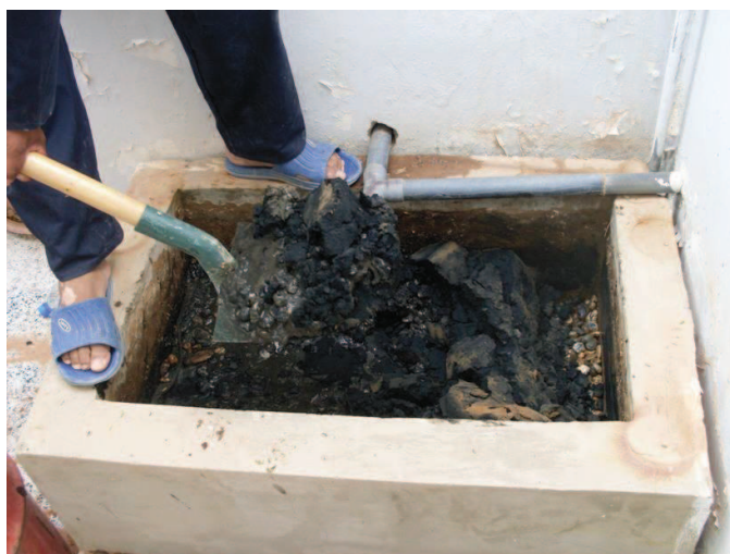
Fig. 9: Excavation of the completely clogged filter media in the original (source: AHT GROUP AG, 2011).
