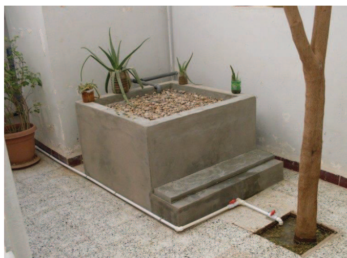
Fig. 10: The rebuilt greywater filter at the project offices in Béni Abbès (source: AHT GROUP AG, 2011).
