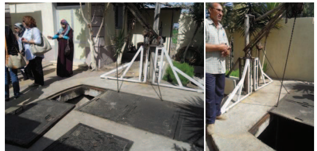
Fig. 7: Pumping station of El-Moufty El-Kobra. On the right picture: Head of the CDA (source: N. Stuber; 2010).
