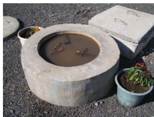
Fig. 8: Area of the top manhole (above biogas fixed dome) of the biogas plant. Clay is used for sealing the lid, and water to keep it wet and thus detect leakages that would show up as bubbles.
