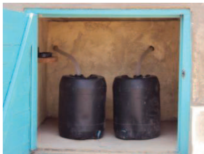
Fig. 11 Two 20 L urine containers with flexible hoses in a vault attached to the UDDT at Mwala Primary School, Ukambani (source: Johannes Orodi, GTZ Kenya, Oct. 2009).
