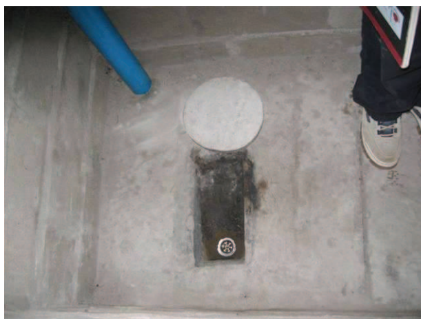
Fig. 5: Inside a new UDDT; the faeces hole is covered with a lid; the urine separation part is fitted with a sieve. You can see the ventilation pipe at the back left (source: M. Fogde, 2003).
