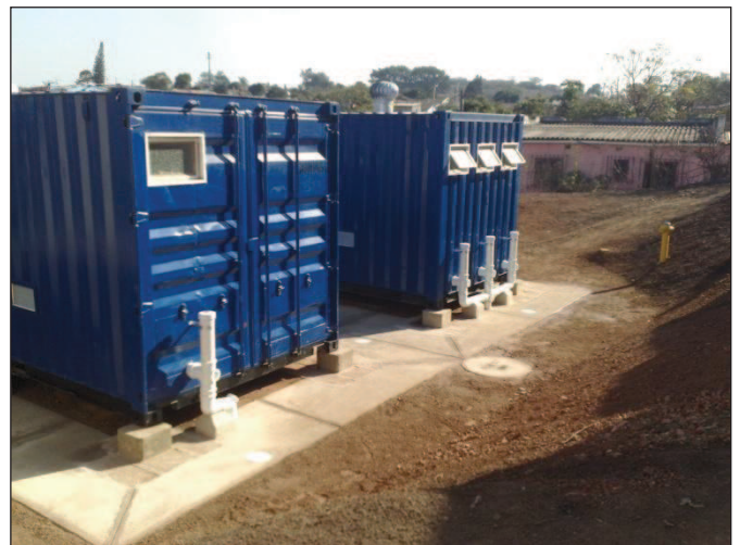
Figure 3: Prefabricated container in Durban (source: eThekweni Water and Sanitation, 2010).
