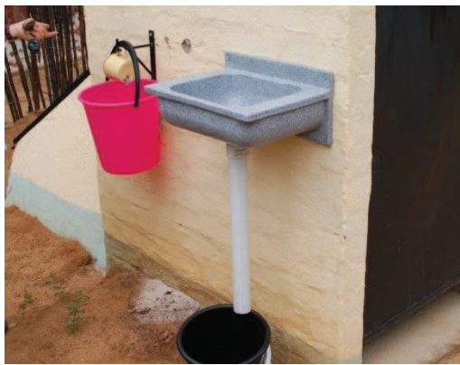
Fig. 6: Basic handwashing facilities attached to the toilets. The pink bucket provides fresh water, the cup is used to fill the basin and the black bucket collects the greywater which can be used for irrigation (source: GIZ, Kleemann, 2011).
