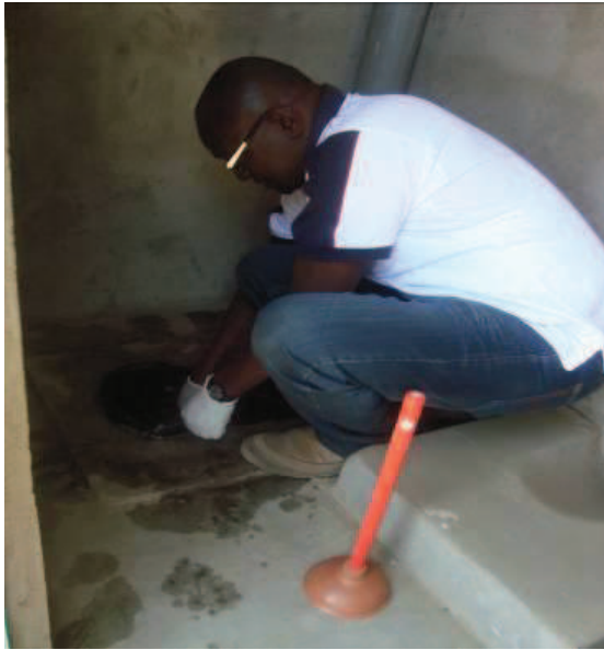
Fig. 8: ROSA project staff unblocking urine pipes at Daraja II primary school UDDT.
