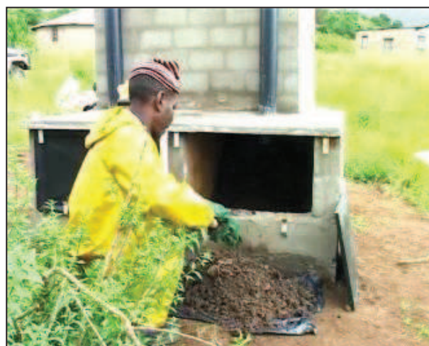
Fig.14: Emptying a UDDT faeces chamber (source: EWS).
