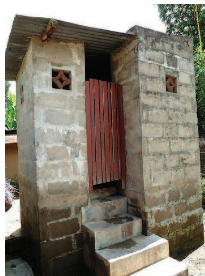
Fig. 3: Well maintained household UDDT in Guara-Guara 8 years after construction (source: A. Leitner, 2011).
