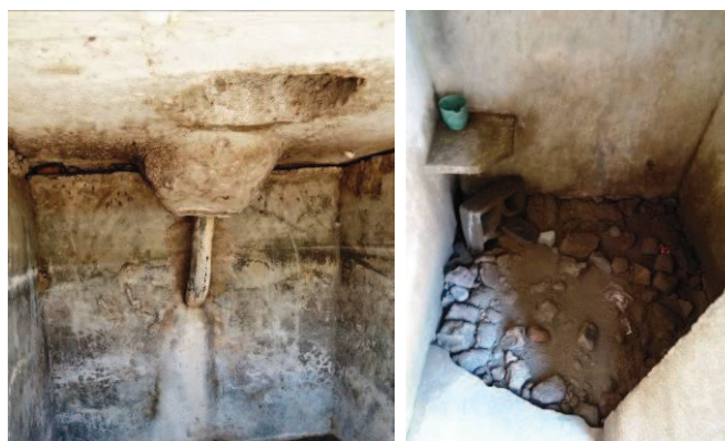
Fig. 9: Situation 8 years after construction: Left: walls of faeces vault with deep cracks. Right: bathing cubicle's concrete floor is broken (source: A. Leitner, 2011).
