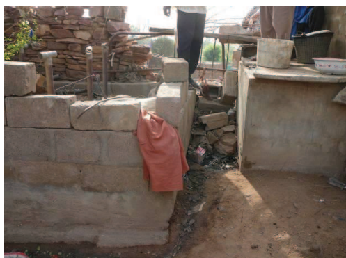
Fig. 4: The same location as Fig. 3: greywater garden on the left side with leaking water from broken pipe (source: Stefan
