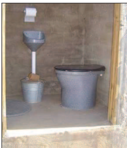
Fig. 11: Inside view of UDDT: urinal for men (left), bucket containing sand or ash, cover over second vault on the left side and urine diversion pedestal on the right (source: EWS).
