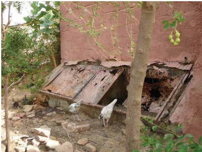
Fig. 9: Rusted iron covers of faeces chambers are falling apart, - no more drying of faeces is therefore possible (source: Stefan Hofstetter, March 2009).
