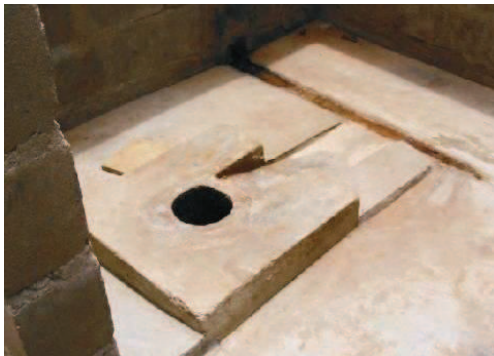
Fig. 6: Latrine urine-diversion squatting pan, where urine drains away to the drainage at the right (source: GTZ, 2002).
