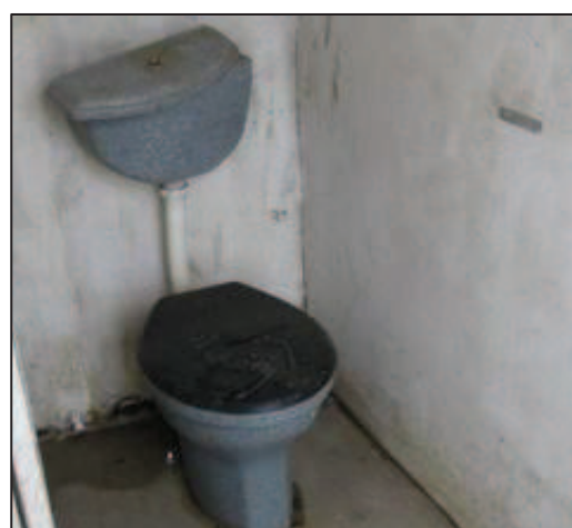
Figure 10: Flush toilet in CAB (source: Roma, 2010).
