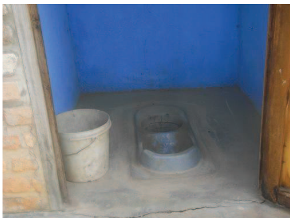
Fig. 9: Inside view of UDDTs at Kiruhura primary school showing plastic urine diversion squatting pan and bucket with ash for covering faeces after defecation. Toilet has been in use for 2.5 years.
