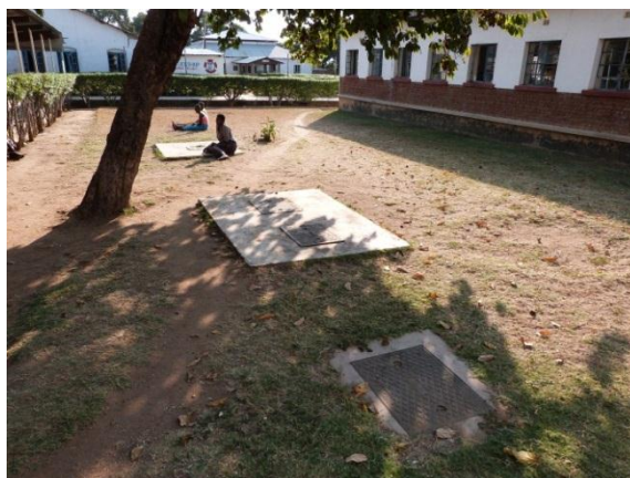
Figure 5.2 – Septic tank (ST6) with soak pit in the background. © Mirco Keller.
