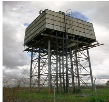
Figure 2. Overhead tanks for the 3-D project
