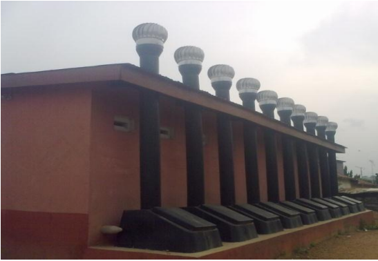
Figure 9. Back view of Enviro - Loo toilet facility
