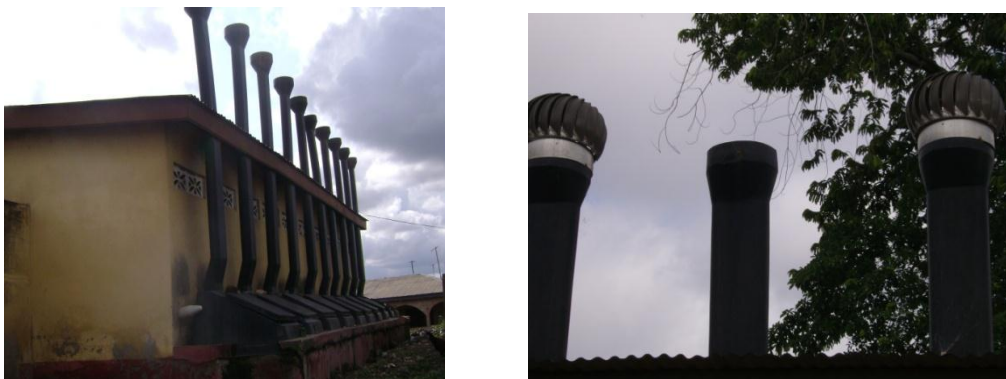
Figure 10. Enviro-Loo with defective components
