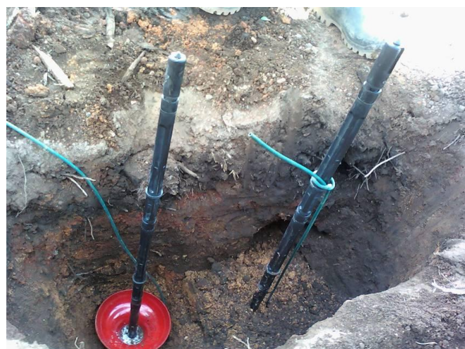
Figure 6.14 Installation of a pair of wetting front detectors at depths of 400mm depth (left) and 1m (right)
