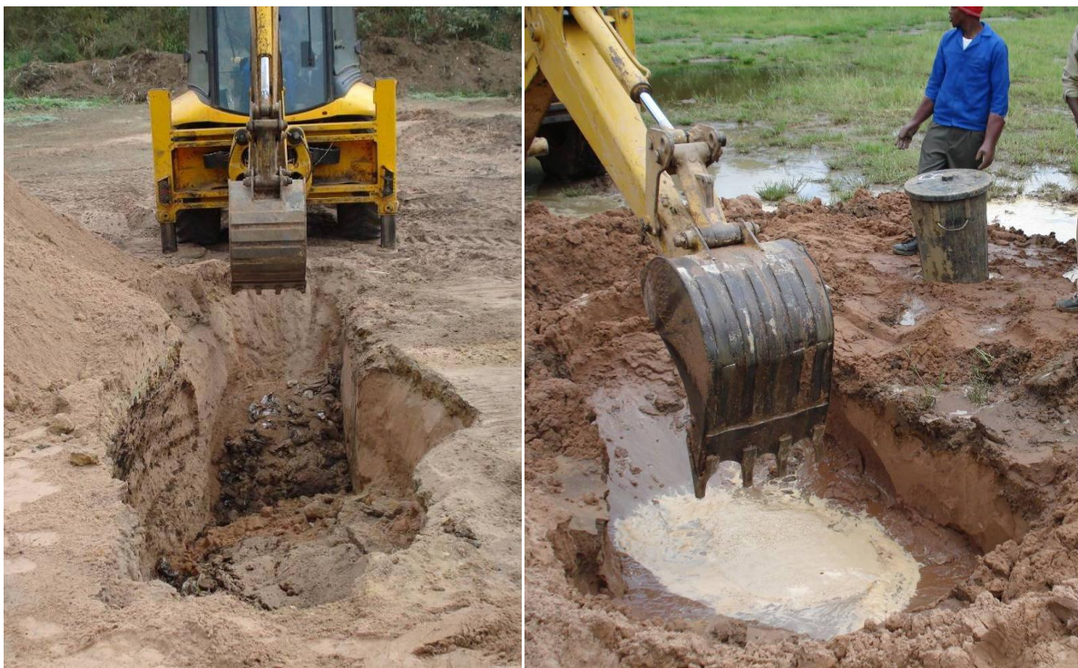
Figure 5.13 Variable conditions resulting in variable pit dimensions
