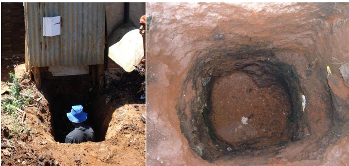
Figure 5.691 Manual excavation of a pit. Start of the sludge layer clearly visible 1.65m below the surface.
