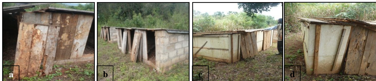
Figure 17: Dilapidated compost chambers
