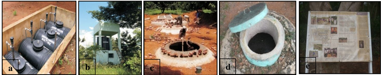
Figure 21: urine storage tanks at sanitary block (a), tank for greywater at the VVU farms (b), biogas digester at time of construction (c), biogas digester at time of field study (d) Sign post (e)
