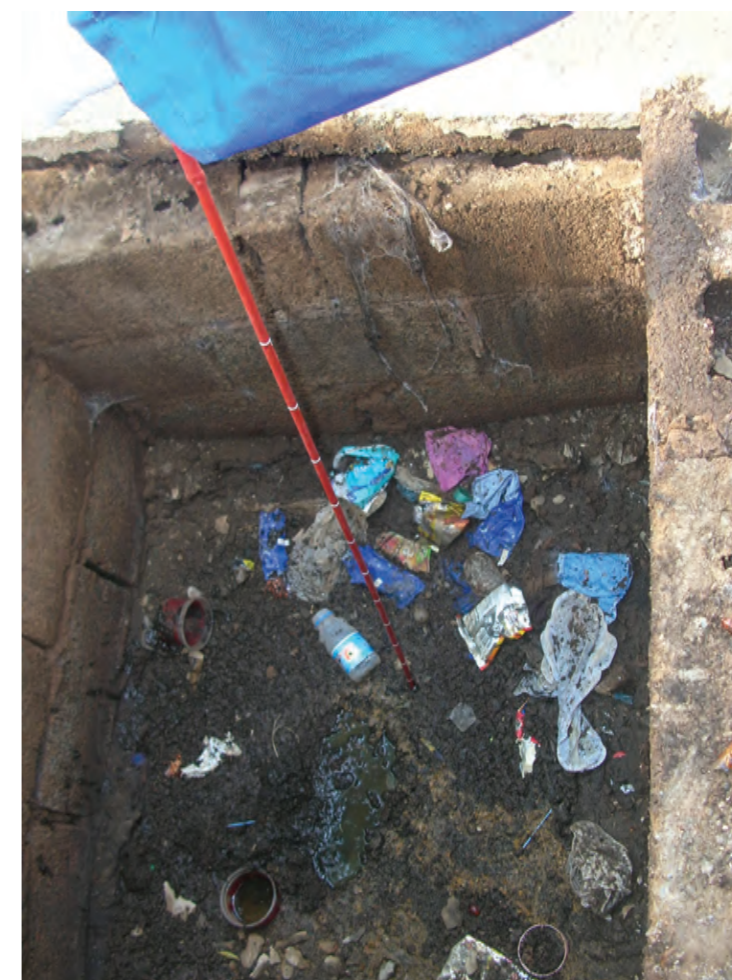
FIGURE 1 Sludge heap under pedestal (pedestal positioned over top of image)
