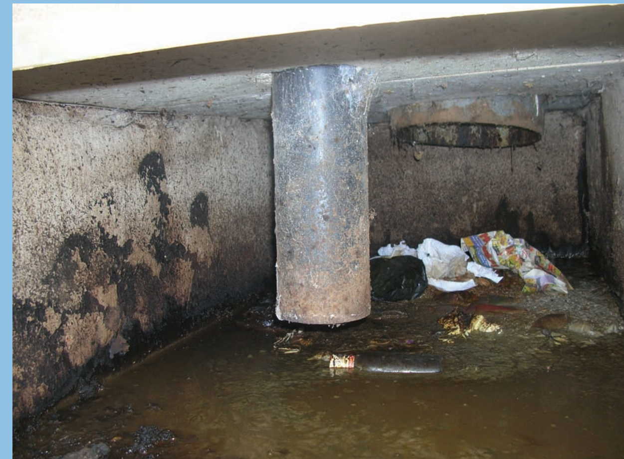
UD active vault
