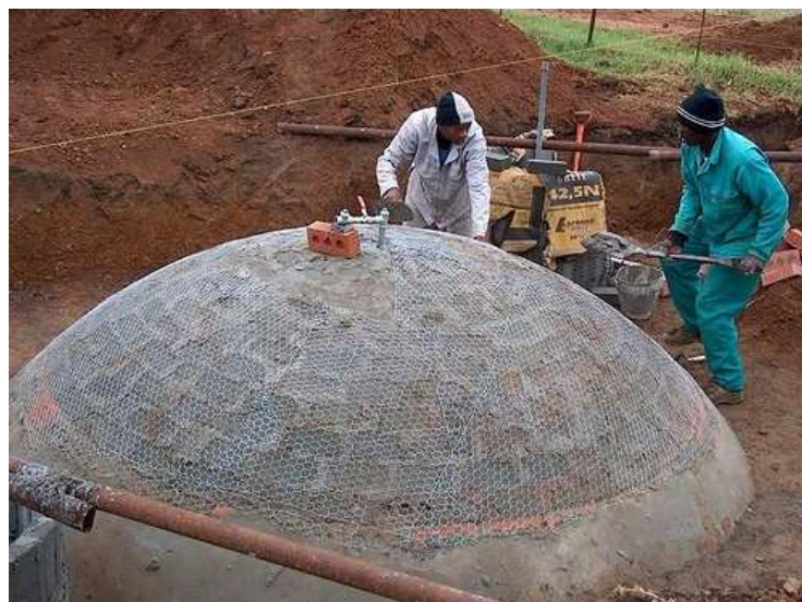
Figure 6.4 Anaerobic biogas reactor built in Lesotho by GTZ (Lepofa, 2006)
