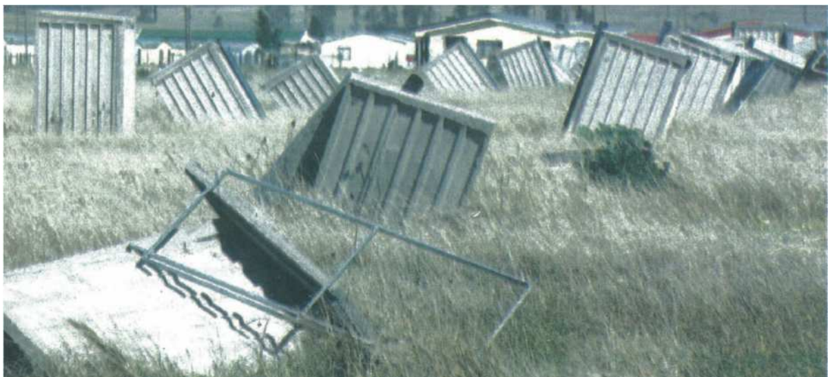
Figure 7.2 Precast VIPs erected at Dutywa in the Eastern Cape which have collapsed due to inadequate foundation preparation
