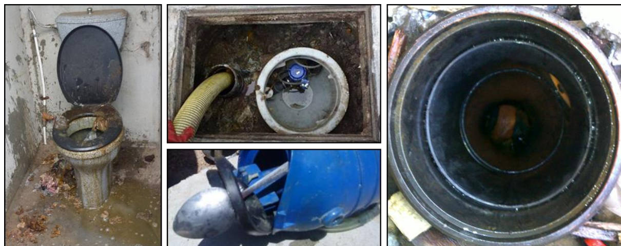
Figure 1. Clockwise from left to right: Typical conditions of a vacuum system toilet; raw sewage being pumped out of a clogged sump and flooded concrete ring; a brick in a sump; and a spoon piercing an interface valve diaphragm.
